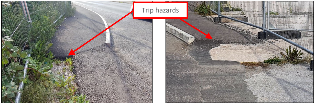
Photo 3.3-1: Western radius is in a state that presents a trip hazard
