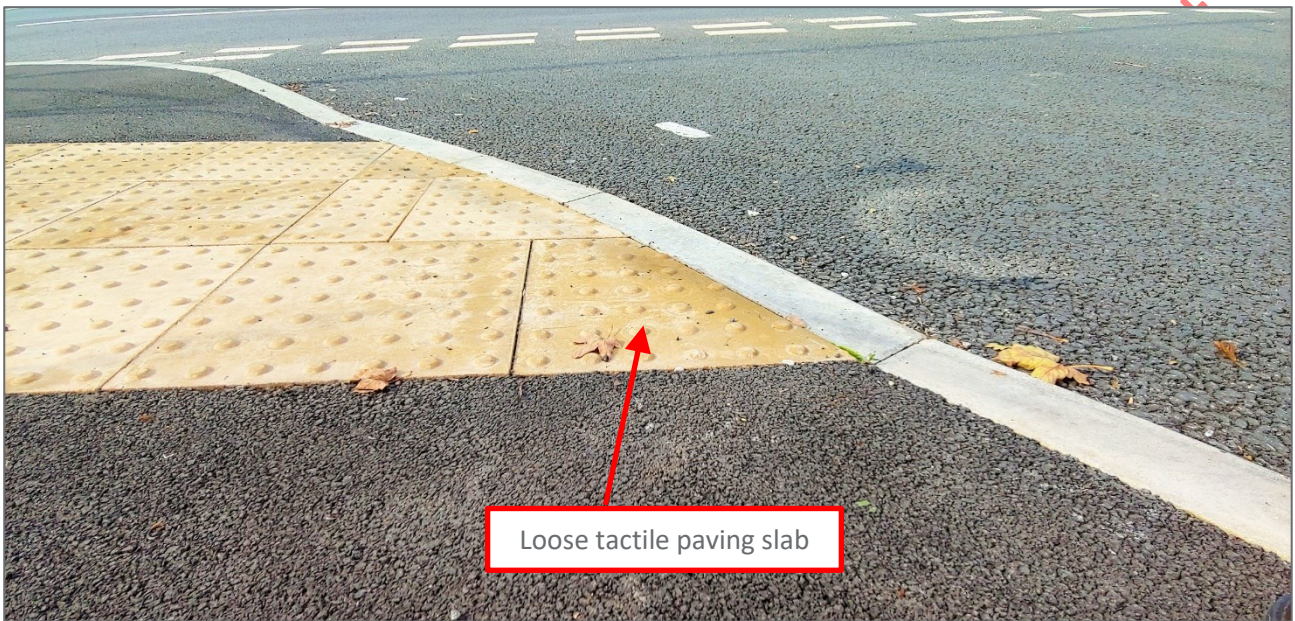
Photo 3.7-1: Loose tactile paving slab will become a slip, trip and fall hazard over a period of time
