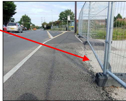
Photo 3.4-2: Footway area with trip hazard at the rear edge – facing east
