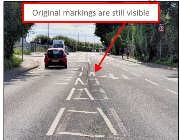
Photo 3.5-2: Original white lining showing through - westbound
