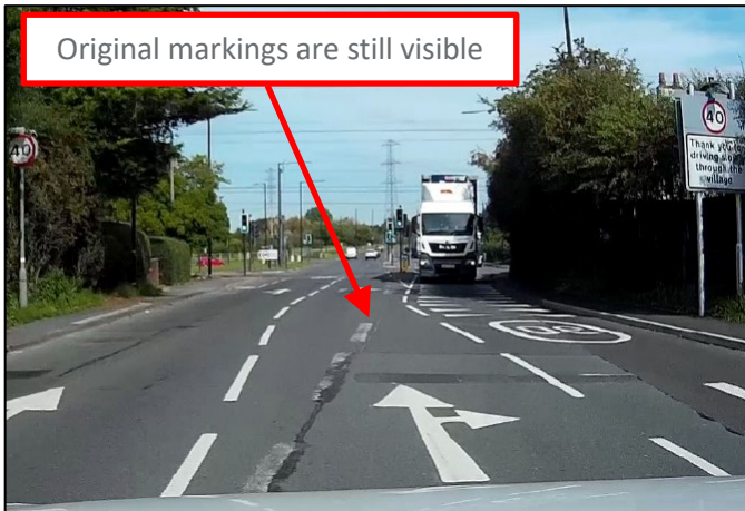
Photo 3.5-1: Original white lining showing through - eastbound
